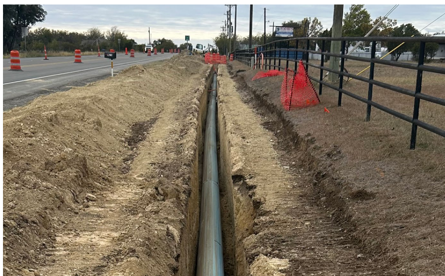
Transmission Line for 536 Well Field, City of Stephenville, Texas
